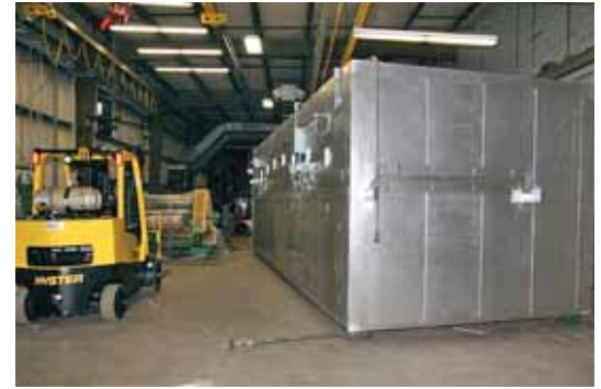
D-P's state-of-the-art, multi-zone dryer just prior to installation
